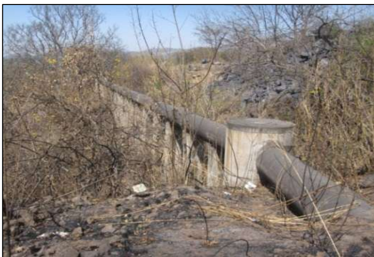
Figure 2: Water pipeline running along the contour of the ridge, parallel to Kanyamazane Road
