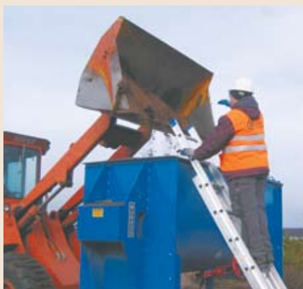
Contaminated soil remediation project site in the remote wilderness of Quebec, Canada
